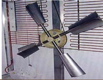
Radiator and fan inside the setter
